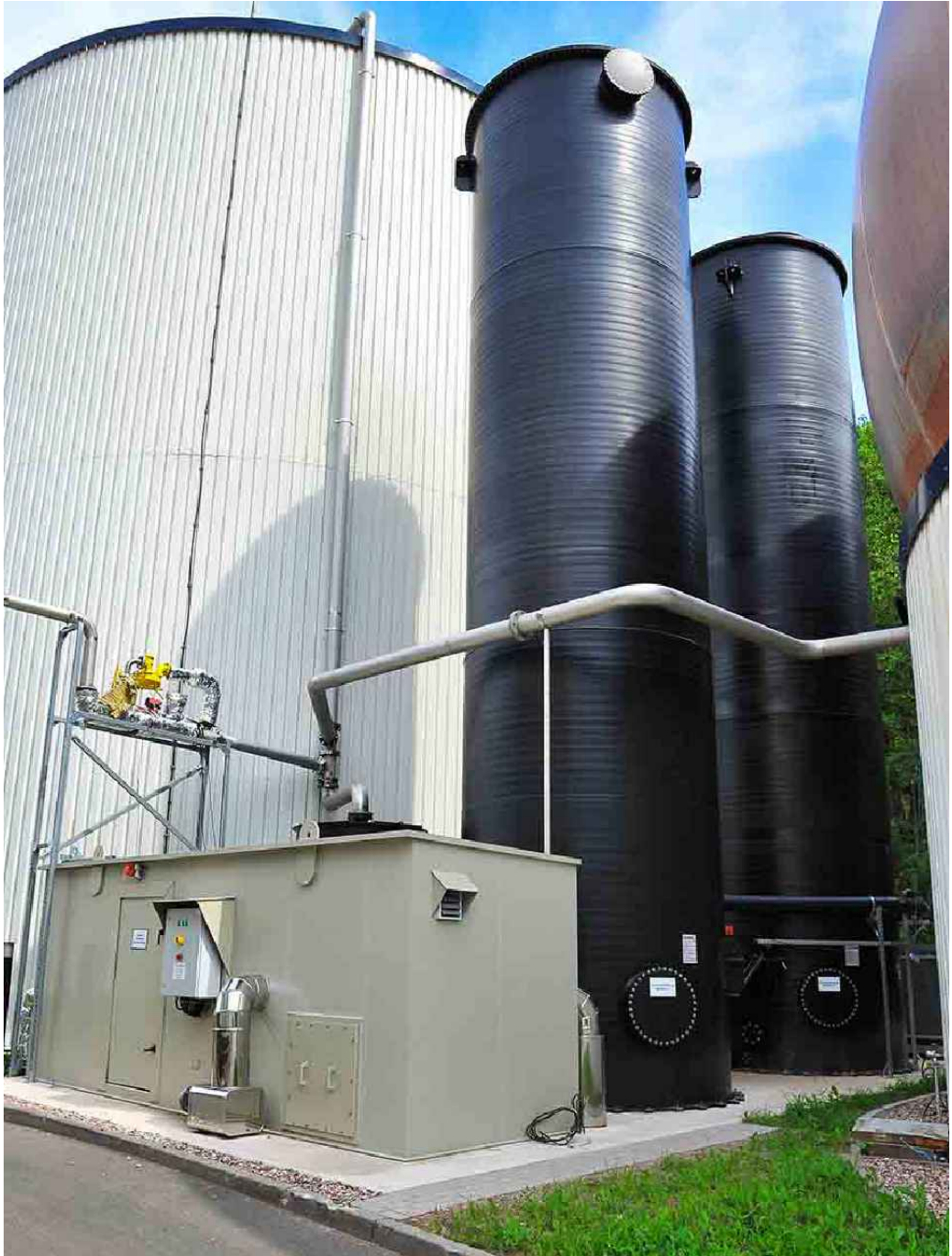
TYPICAL DE-SULPHURISATION TANKS (N.T.S.) (CONTROL CONTAINER FOREGROUND, 2 No. HDPE FILTRATION TOWERS)
